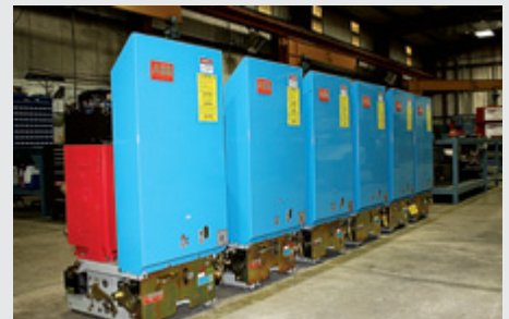
Remanufactured breakers from Circuit Breaker Sales & Co., Inc. helped keep a utility in the Northeast up and running during Superstorm Sandy.
